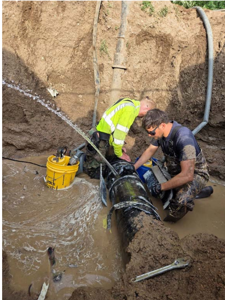
Figure 3. Repair clamp installation on a live water main break performed by 633 Construction in 2025.
