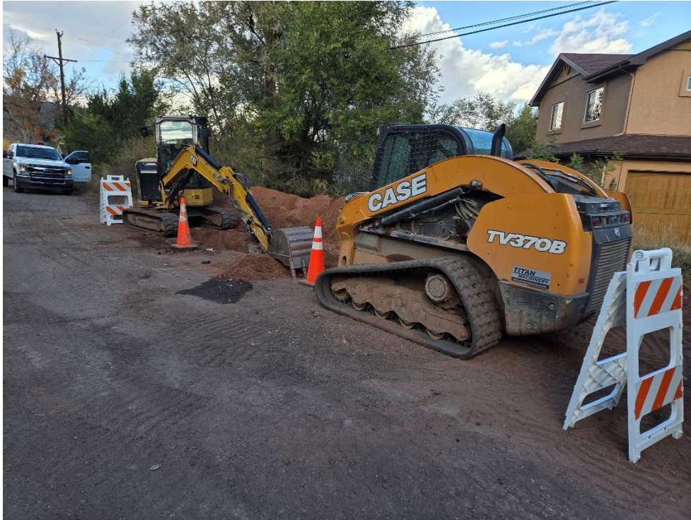
Figure 1. 633 Construction completing a semi-emergency storm sewer installation project for the City of Manitou Springs in 2025.
