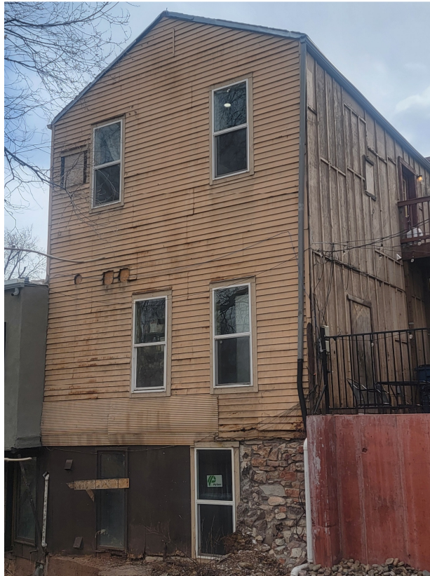
Showing deteriorating siding & trim
