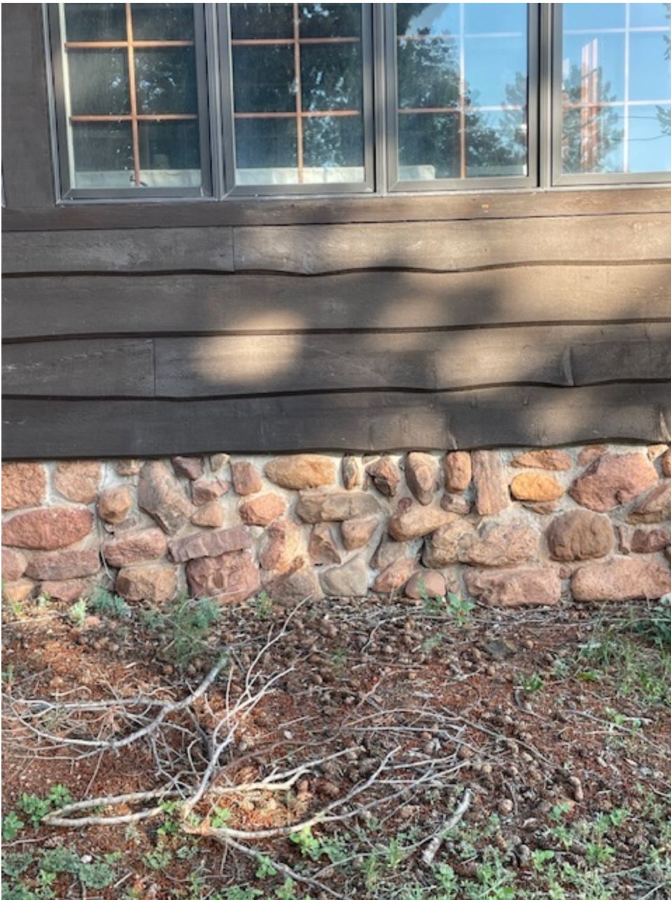
Neighbor porch enclosure with natural stone foundation and faux divided lites in windows. Sent from my iPhone
