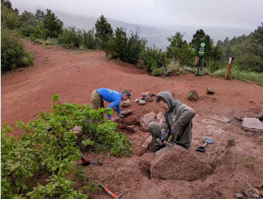
Figure 6: RMFI crew building a rock armored ramp at the top of the trail reroute.
