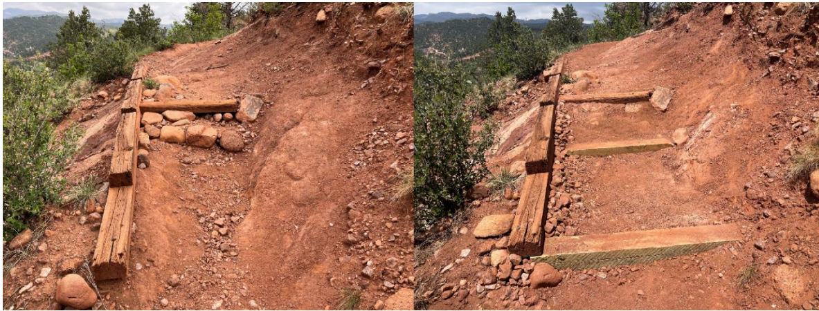
Figure 8: Before (left) and after (right) A failing timber structure rebuilt on Intemann Trail.
