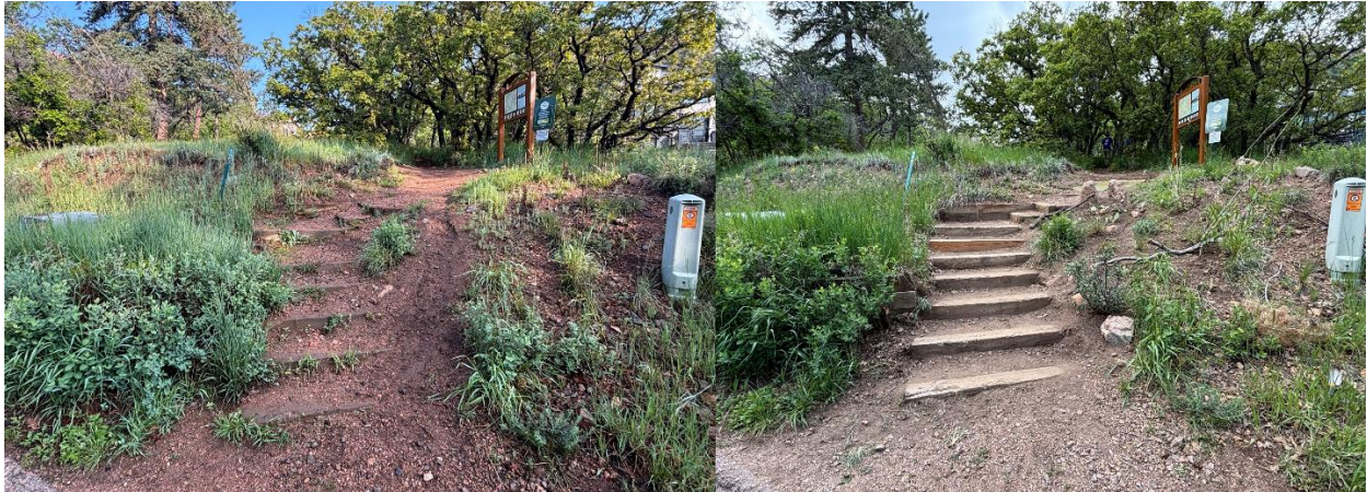
Figure 11: Before (left) and after (right) of trailhead steps repaired at Intemann Trailhead.
