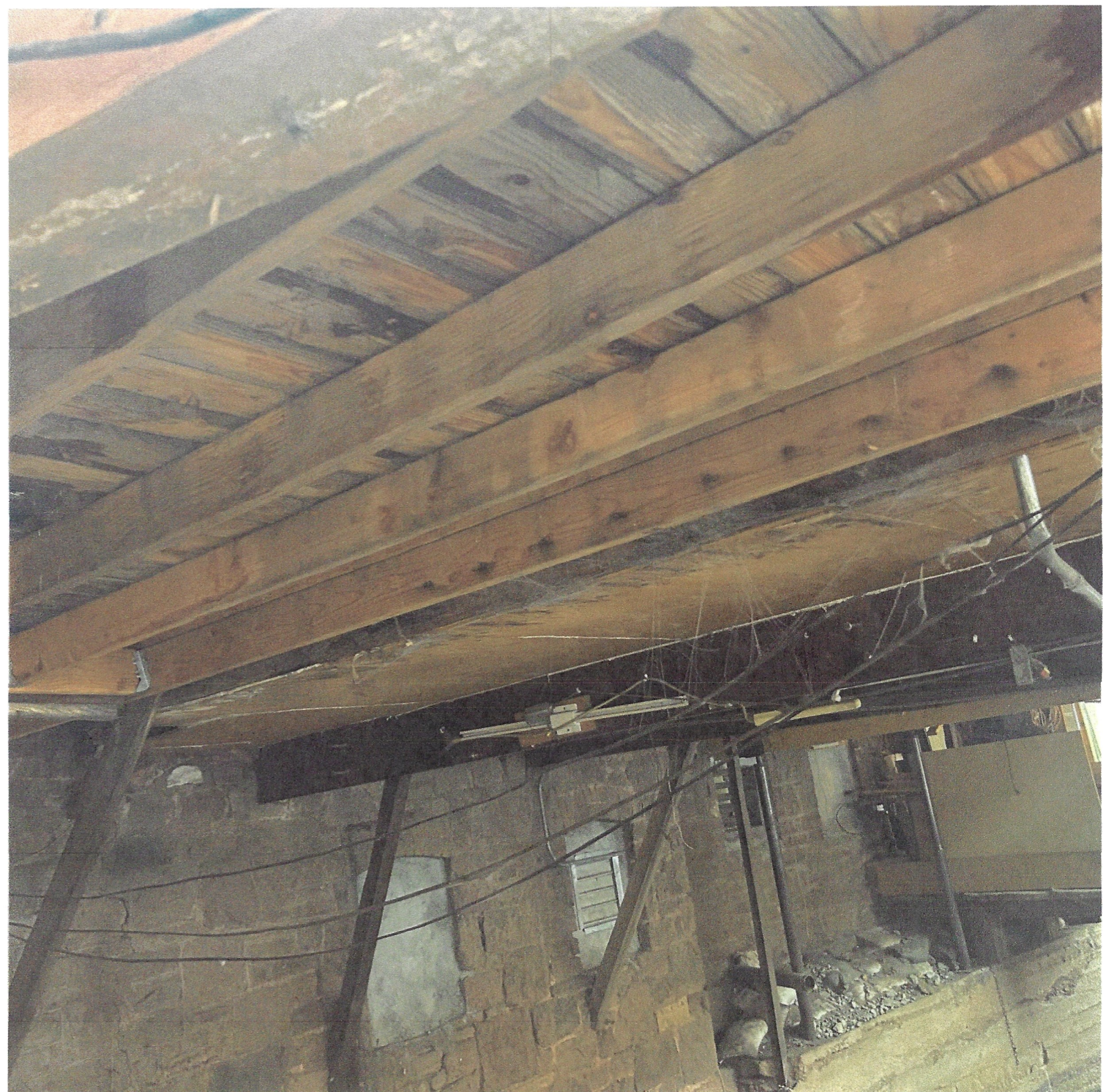
BOWING AND OVERSPAN JOIST
