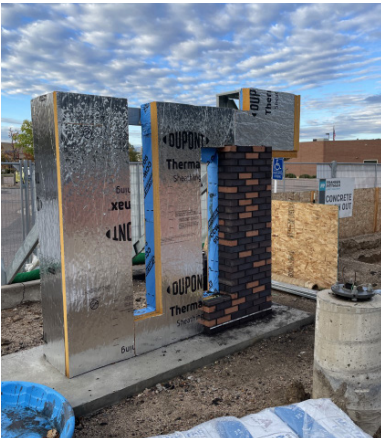
Mock-ups of building systems onsite ensure specifications and standards.
